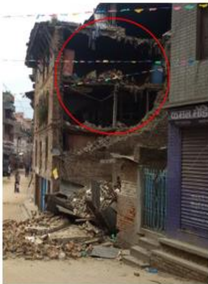
Fig. 4.c: Out of plane failure
