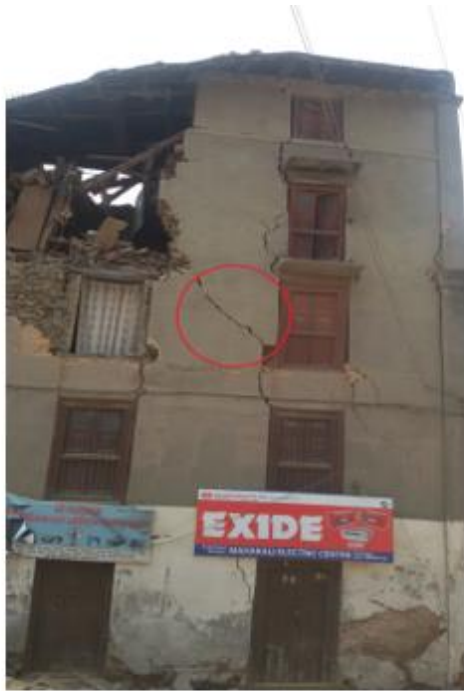
Fig. 1.a: Diagonal shear crack
