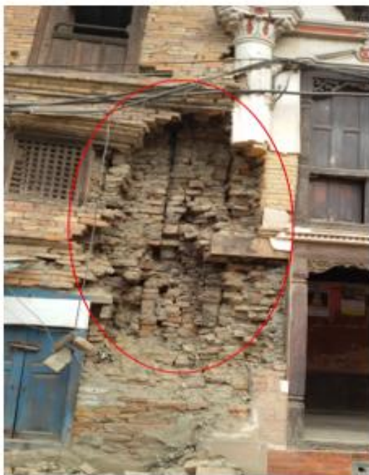
Fig. 6.c: Failure of outer layer of brick
