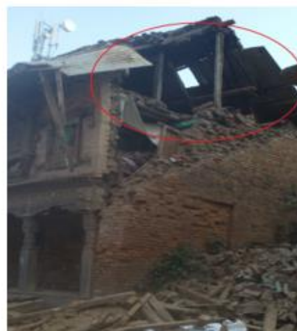
Fig. 5.d: Gable roof wall failure
