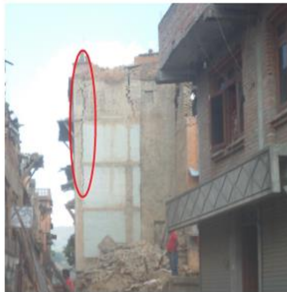
Fig. 3.d: Vertical crack at corner
