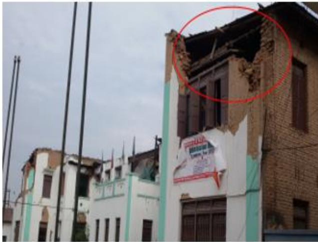
Fig. 5.a: Top roof wall failure
