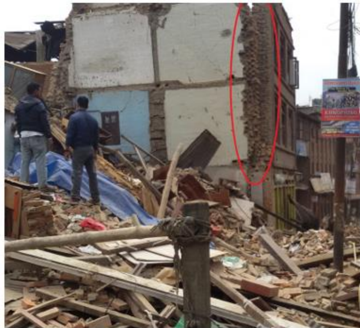
Fig. 2d: Corner failure
