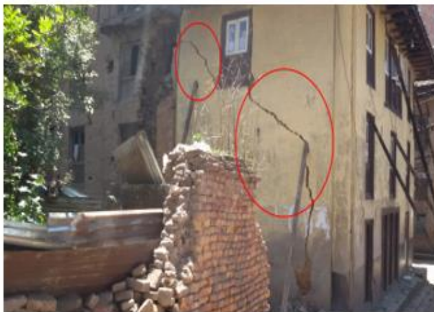
Fig. 1.c: Diagonal shear crack
