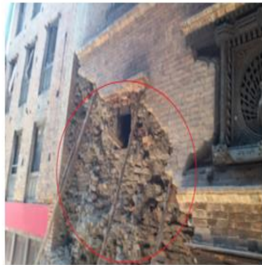
Fig. 6.b: Failure of outer layer of brick wall
