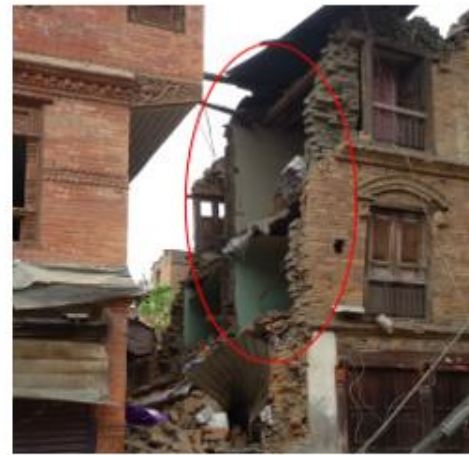
Fig. 4.b: Out of plane failure
