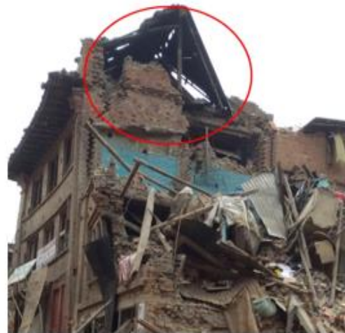
Fig. 5.b: Gable roof wall failure
