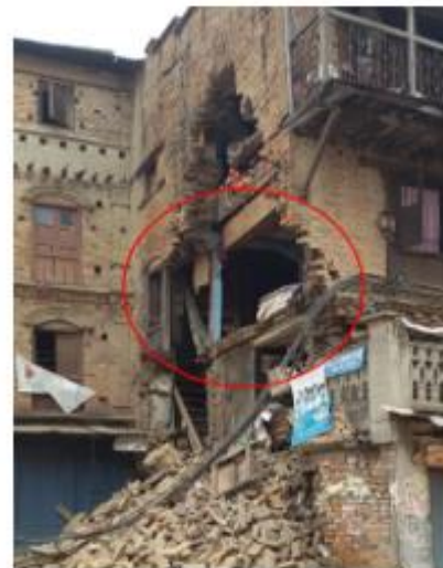
Fig. 4.d: Out of plane failure in lower stories
