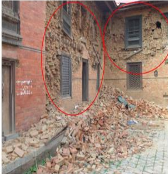
Fig. 6.a: Failure of outer layer of brick wall
