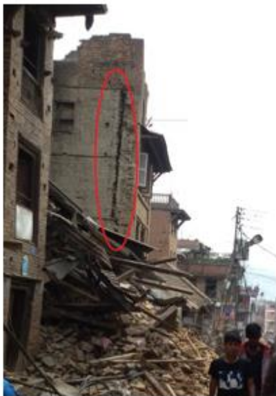
Fig. 3.c: Vertical crack at corner
