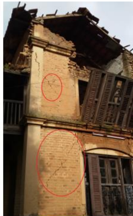
Fig. 1.b: Diagonal shear crack
