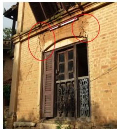
Fig. 1.d: Vertical shear crack
