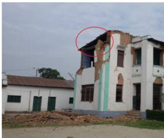
Fig. 5.c: Top roof wall failure
