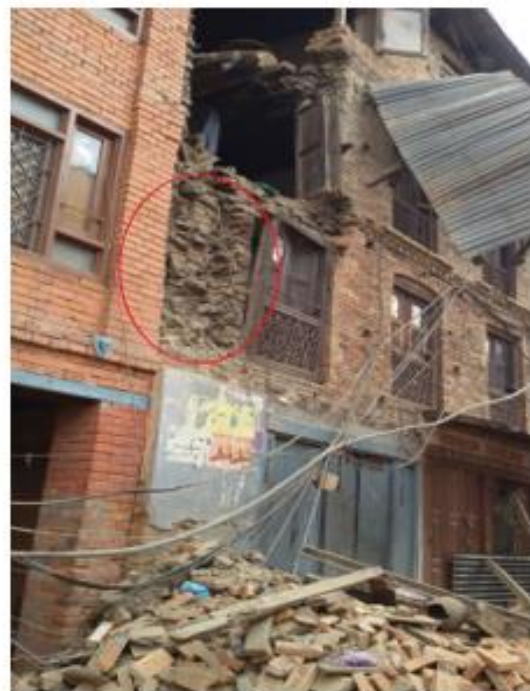
Fig. 6.d: Failure of outer layer of brick
